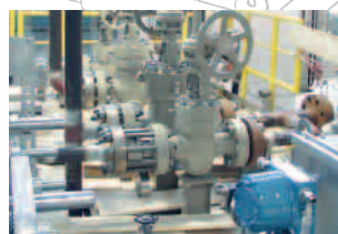
Methanol injection units for North Sea offshore applications. Capacity 2 x 45 m 3 /h Discharge pressure 370 bar Power installed 2 x 570 kW
