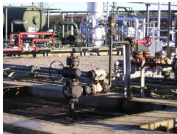
Figure 3 Pump System, Storrington
